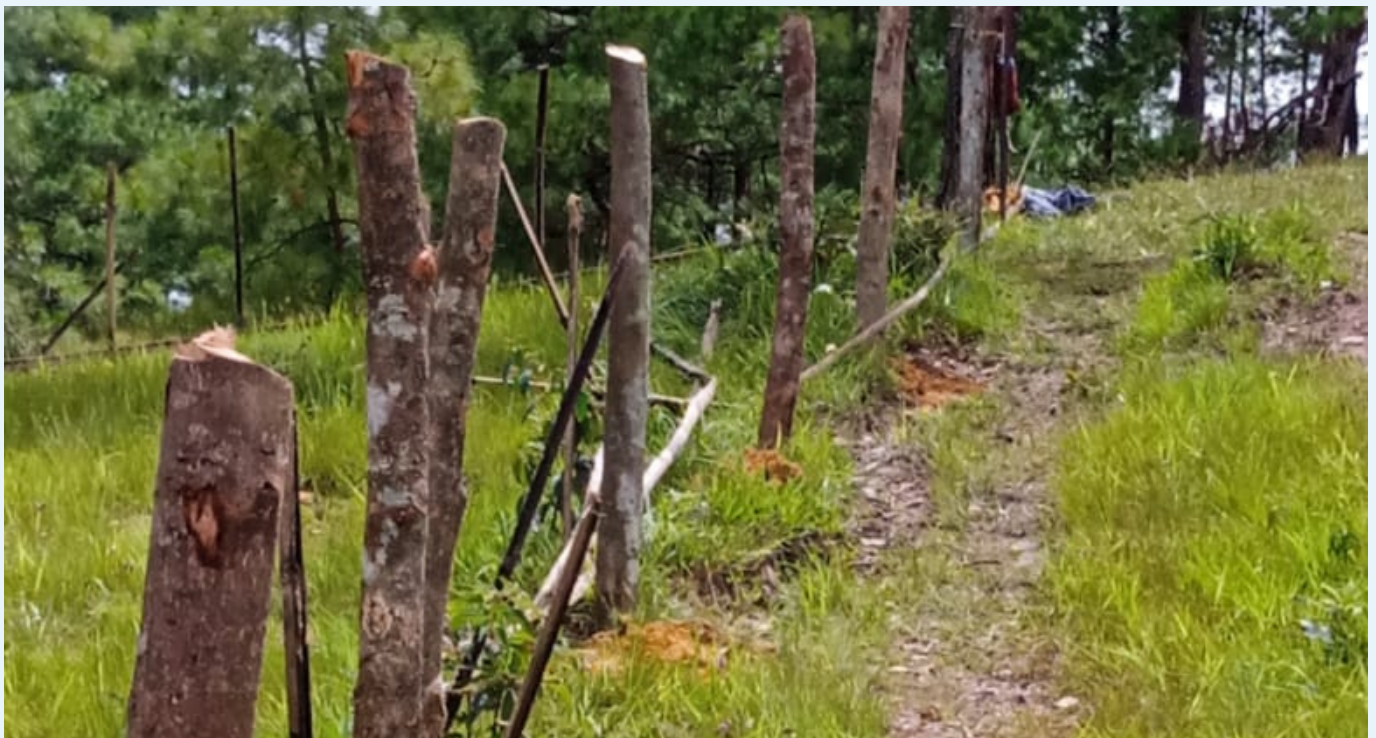
The installation of poles surrounding the plantation area in Pomlahier village was successfully completed on July 28, 2023.
